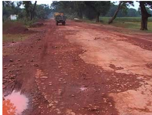
No lane infrastructure
